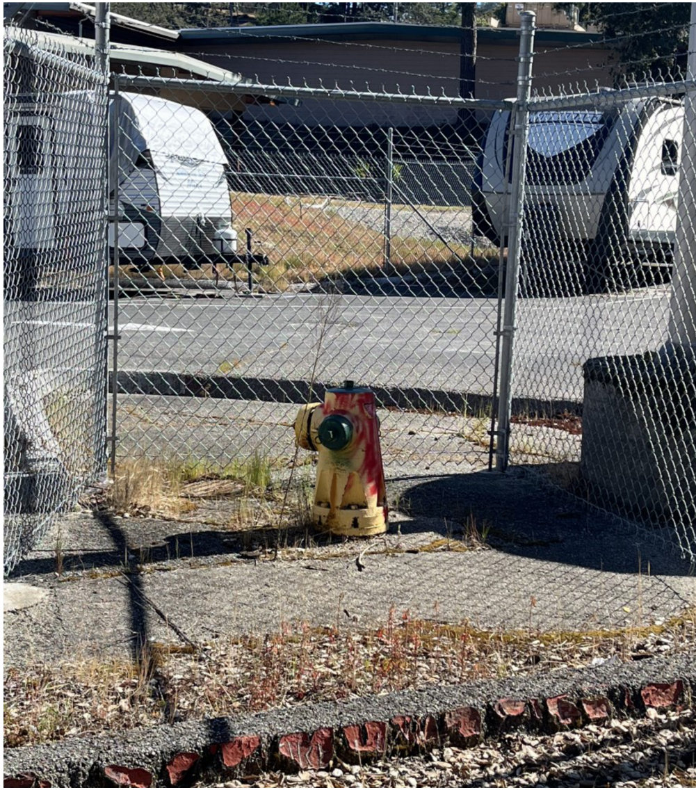
7 EXISTING FIRE HYDRANT NEAR BUILDING 3
