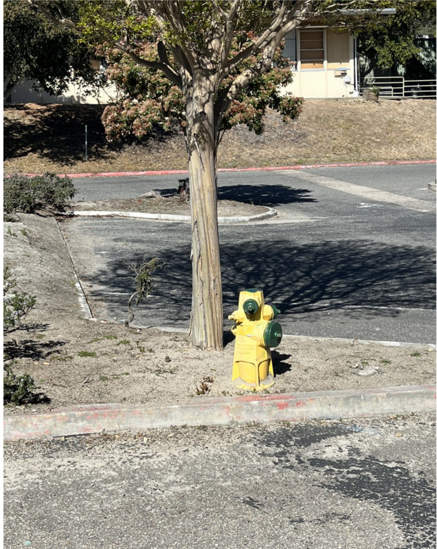
10 EXISTING FIRE HYDRANT NEAR BUILDING 9 (SOUTH)
