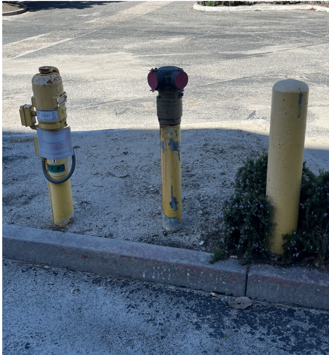
12 EXISTING FIRE DEPARTMENT CONNECTION & PIV BUILDING 9 - WEST (PARKING ISLAND)
