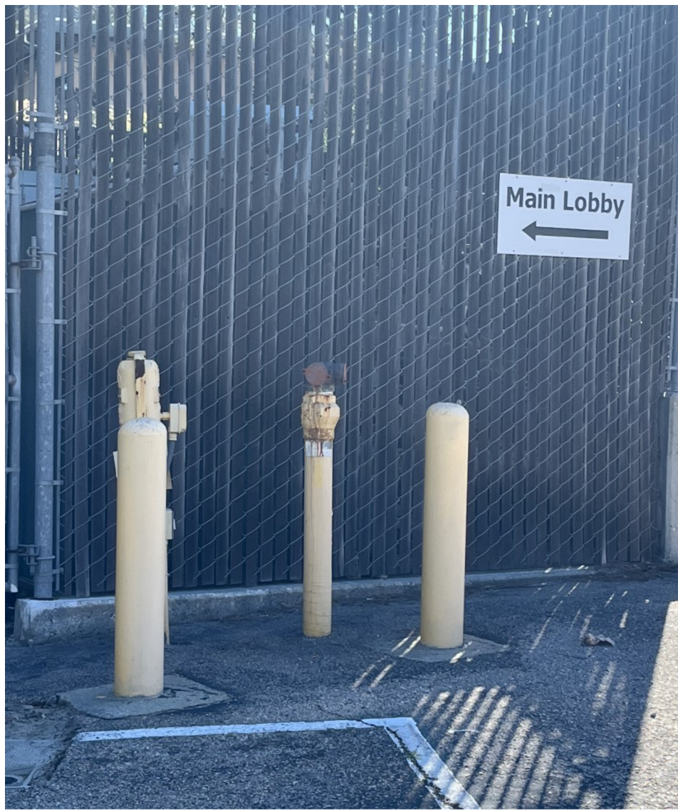
13 EXISTING FIRE DEPARTMENT CONNECTION & PIV BUILDING 9 - SOUTH
