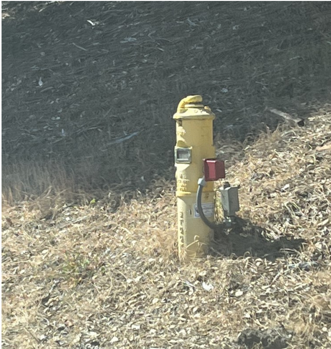
16 EXISTING PRESSURE INDICATOR VALVE BUILDING 1 - EAST (PARKING LOT SIDE)
