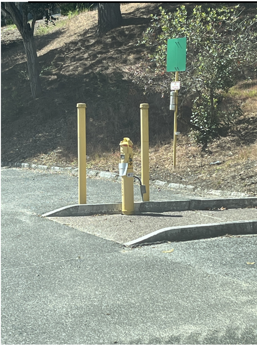
15 EXISTING PRESSURE INDICATOR VALVE BETWEEN BUILDING 1 & 2 - PARKING LOT
