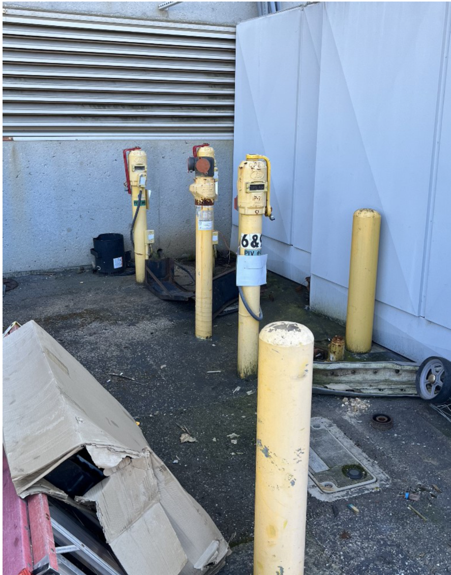
8 EXISTING FIRE DEPARTMENT CONNECTION & PIV'S BUILDING 9 - WEST
