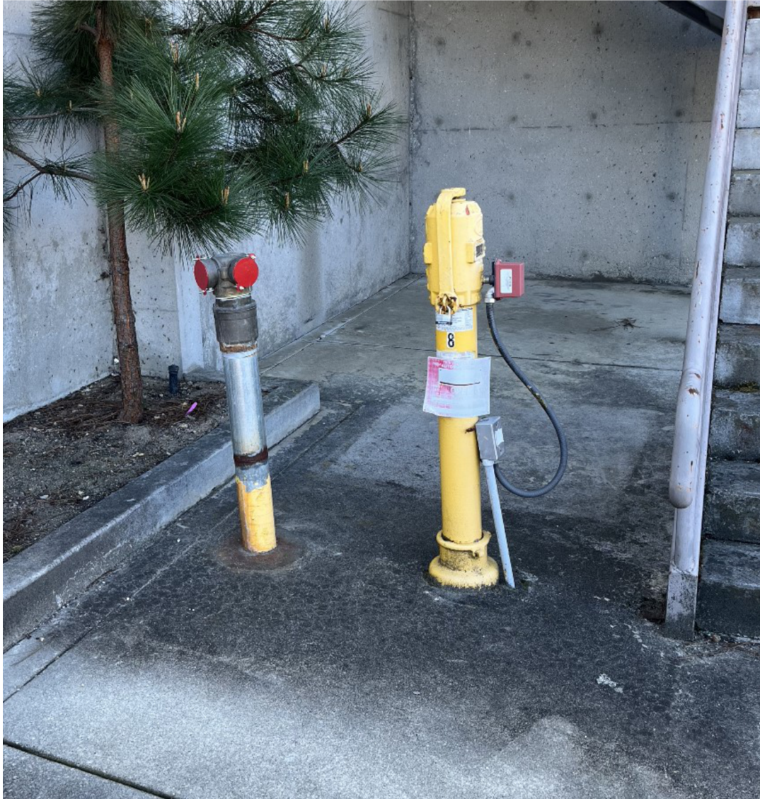
14 EXISTING FIRE DEPARTMENT CONNECTION & PIV BUILDING 9 - NORTH (EXTERIOR STAIR)
