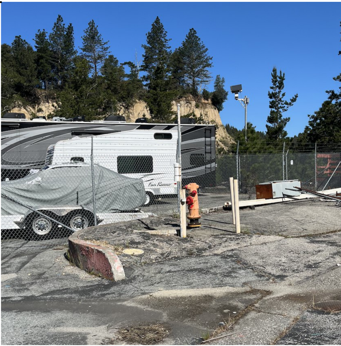
11 EXISTING FIRE HYDRANT NEAR BUILDING 8
