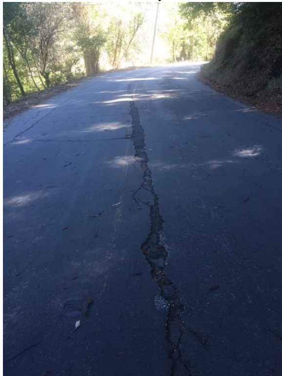
Poor Roadway Condition
