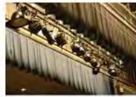
Technical support systems (lighting & sound)
